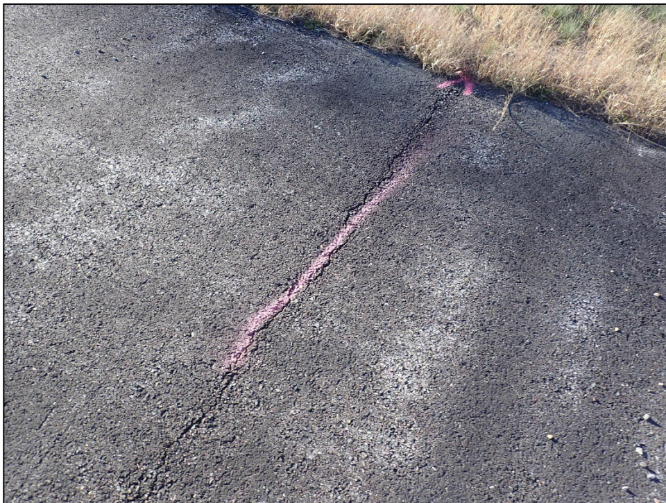
TW-11-15: L&T Cracking
