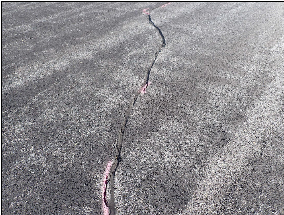
AP-11-10: L&T Cracking
